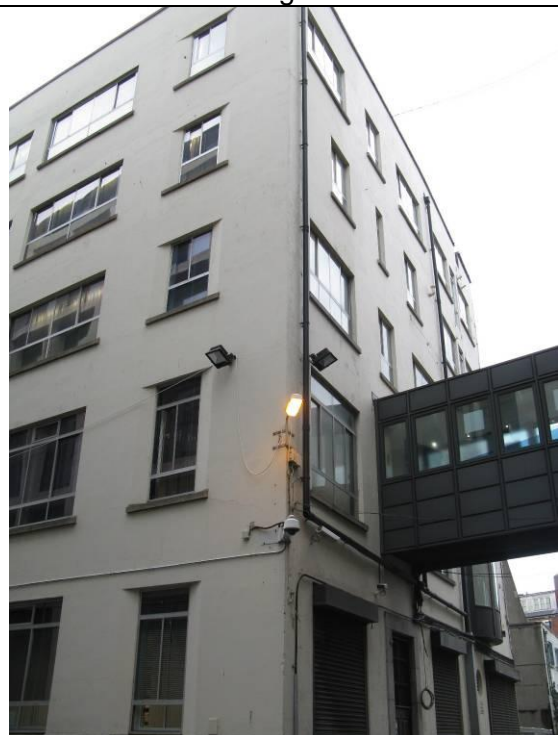
Splayed reveals to portrait window openings bookend the south elevation. Note connecting bridge
